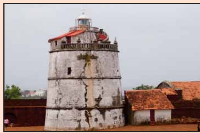
Cracked and old, yet splendid
