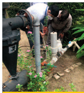
Sprinkler system at AIS Noida
